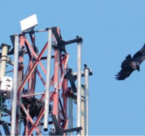
IP backhaul, India
